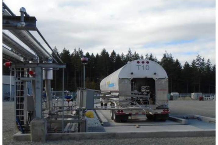
A tractor trailer gets prepared to distribute liquefied natural gas at FortisBC's new trailer loading facility in Ladysmith, British Columbia
